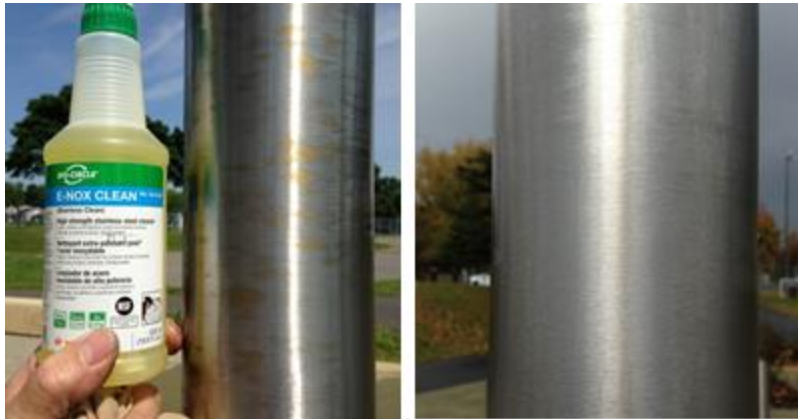
Figure 12: After Cleaning (Left) vs. After E-Nox Clean (Right)
