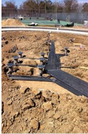
Figure 26: Piping to Feature Bases
