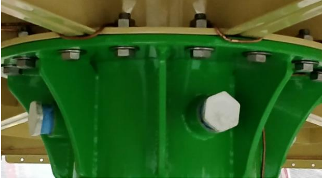
Figure 29: Plugged Upper Ports
