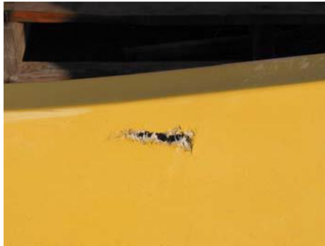
Figure 15: Puncture Holes in FRP
