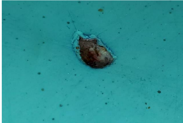
Figure 20: Small Chips in FRP
