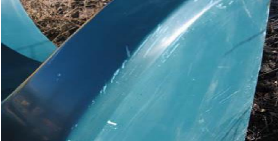
Figure 22: Scratches in Gelcoat
