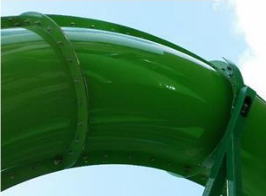
Figure 74: Buffed and Clear Coater Large Repair, Outside
