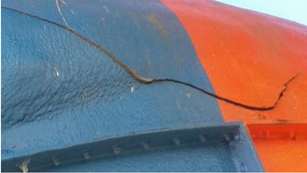
Figure 14: Crack in FRP
