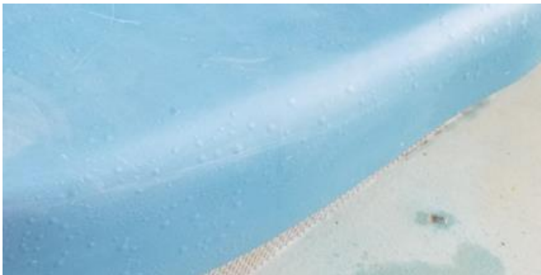
Figure 59: Gelcoat Blisters Needing Barrier Coat
